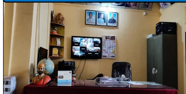
CCTV Setup in Principal Cabin
