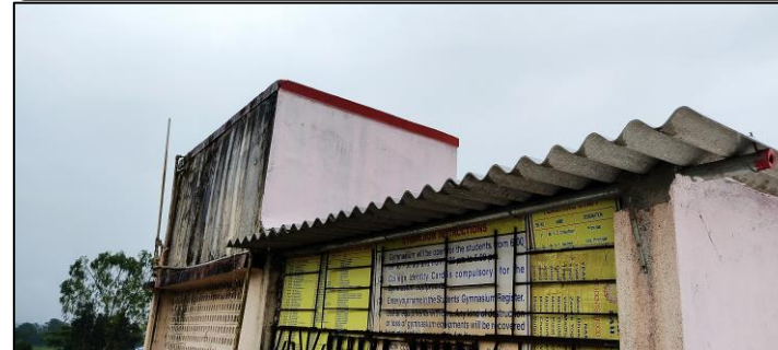
Water Tank on Terrace
