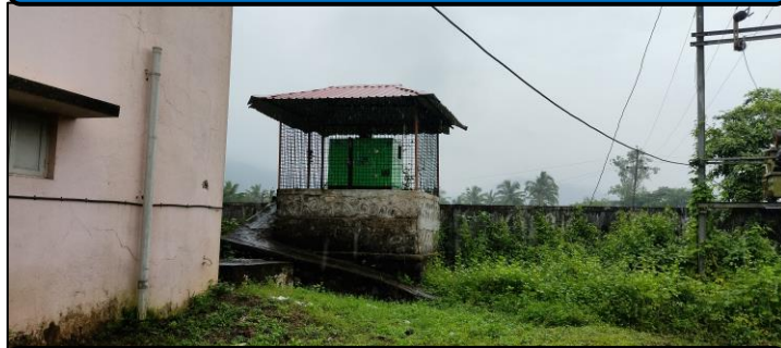
Shade for High Capacity Power Generator
